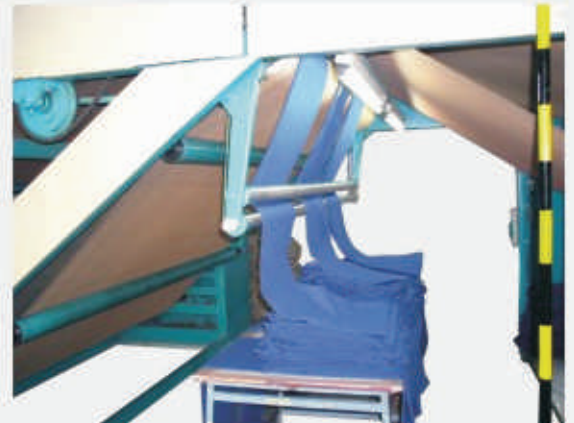
Plaiting unit through conveyor
